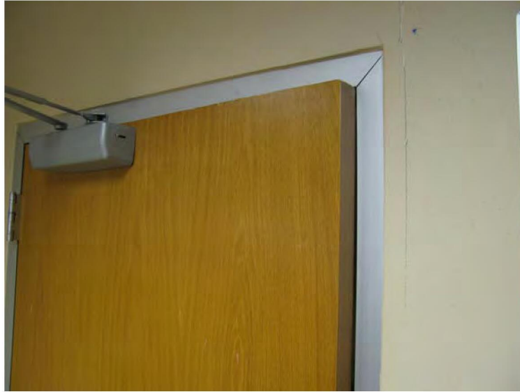
Sticking bathroom door
