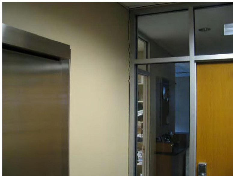
Separation between door frame and dry wall
