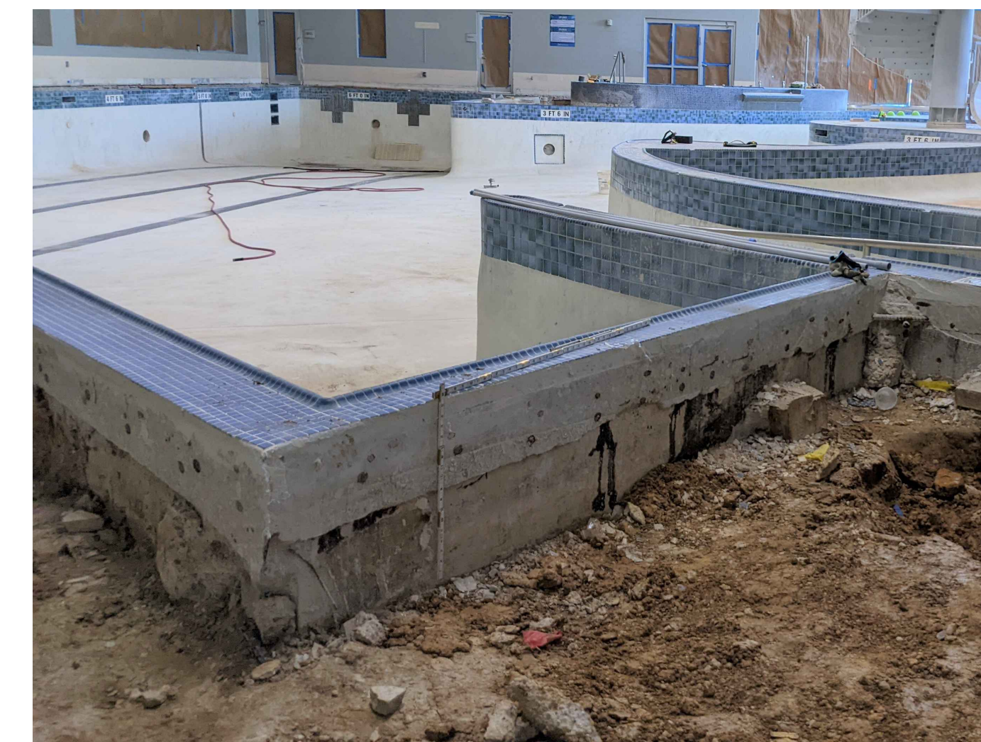
PHOTO 4 - CLOSEUP OF NO BAR STUBS AT EAST POOL WALL, AT STEPS INTO POOL
