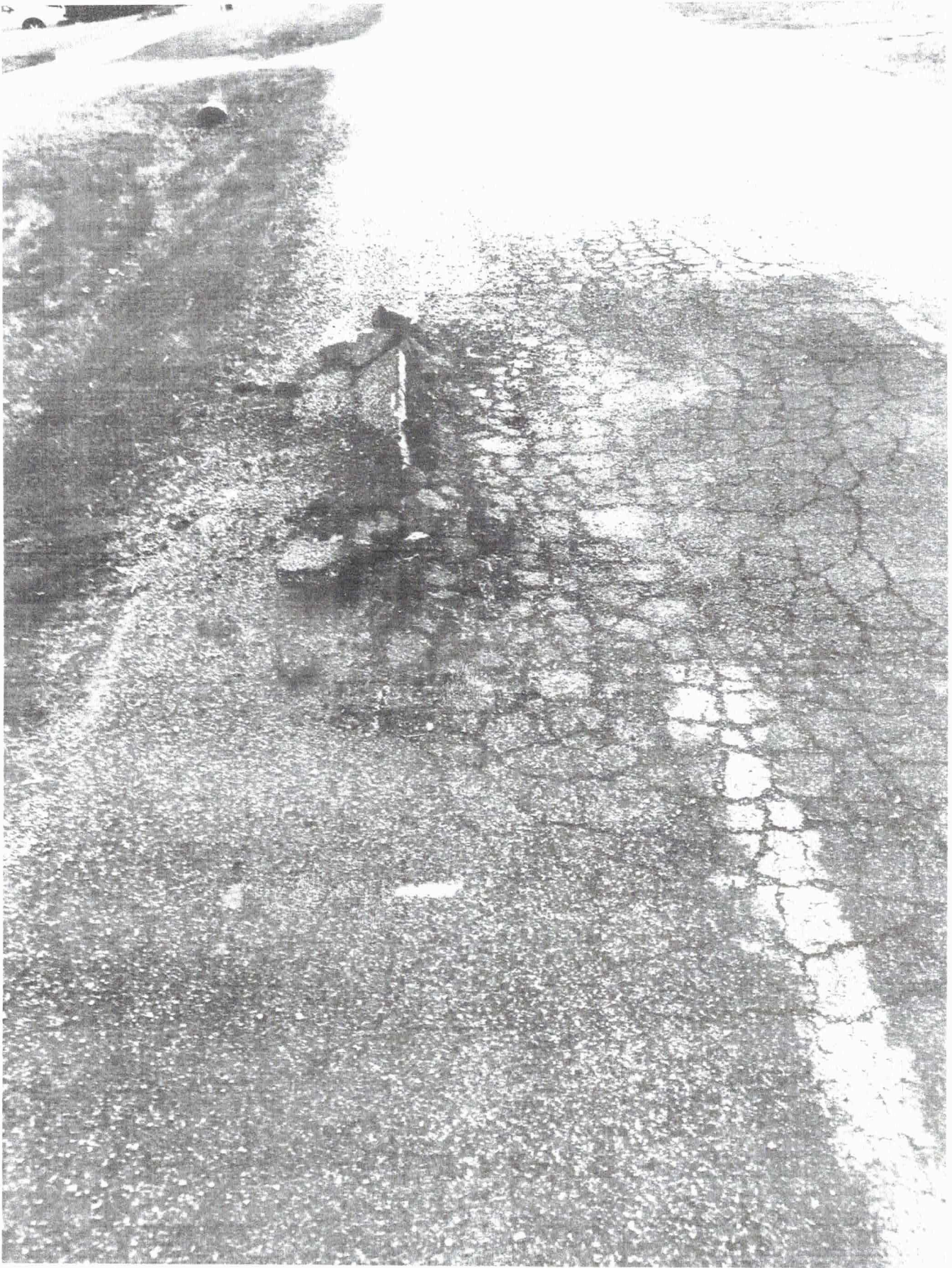
Oakhill Road damage normal traffic
