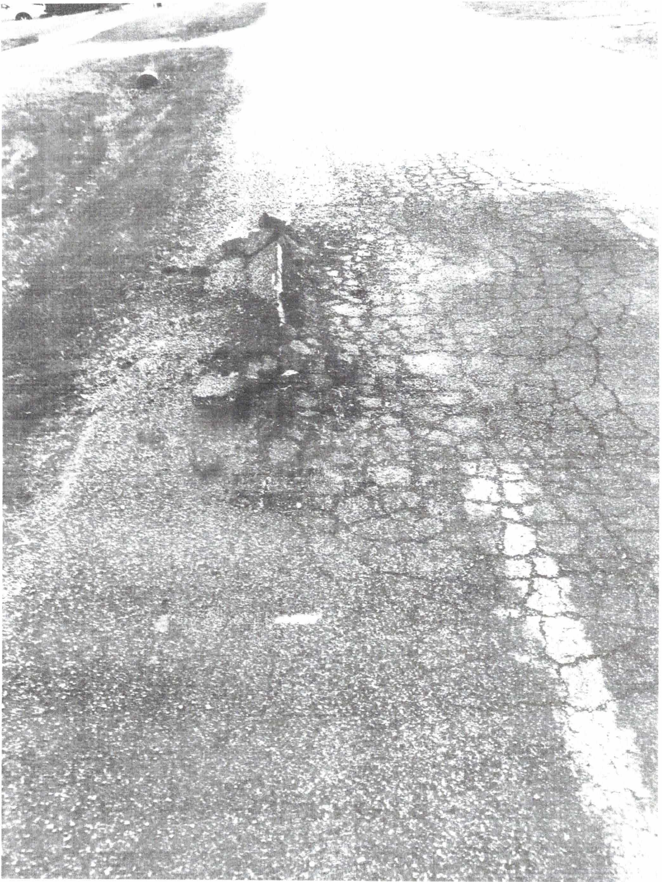
Oakhill Road damage normal traffic
