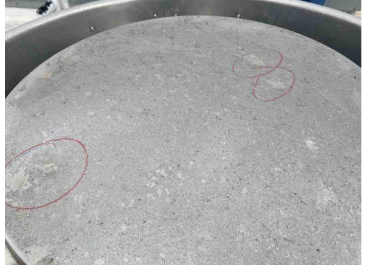
Group: 1.26 - Category: Typical Detail Comments: View of hail strikes on exhaust cap
