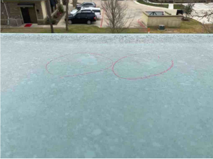
Group: 1.25 - Category: Typical Detail Comments: View of hail strikes on coping
