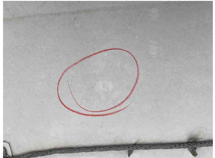
Group: 1.28 - Category: Typical Detail Comments: View of hail strike that did not penetrate roof membrane
