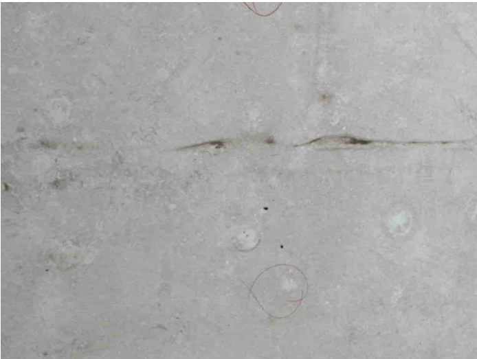
Group: 1.27 - Category: Typical Detail Comments: View of hail strike that did not penetrate roof membrane
