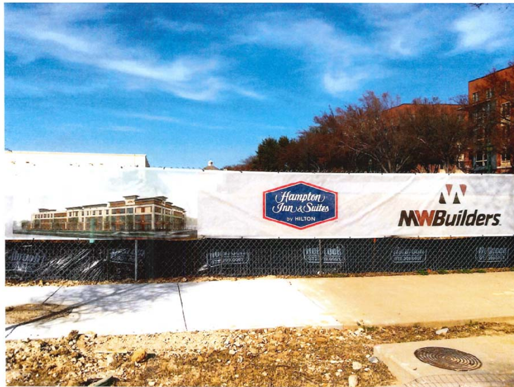
Example of a Fence Wrap on a Non-Residential development currently under construction.
